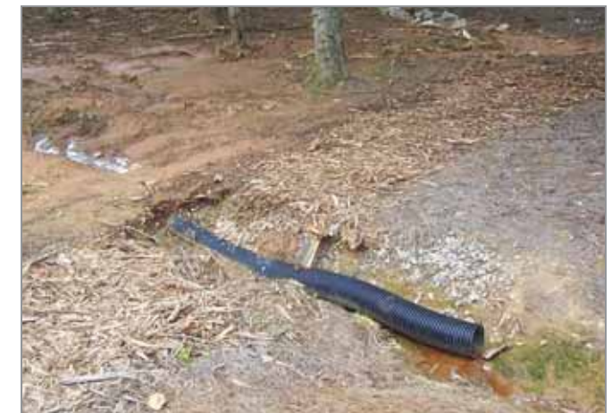
✗ Wood chips can become displaced after rain events, and should not be used for stormwater drainage.
