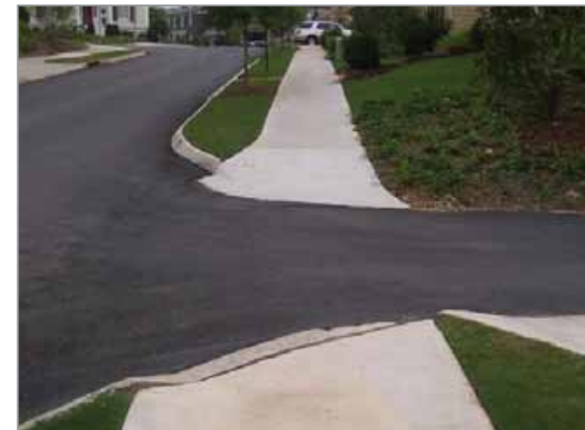
Sidewalk does not continue across alley
