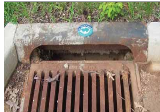
✓ Stenciling raises awareness of the materials that should not enter the storm drain.
